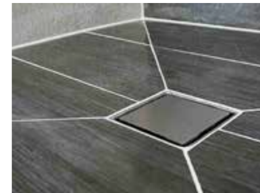
— Floor Waste Tile insert floor waste Location: Bathroom
